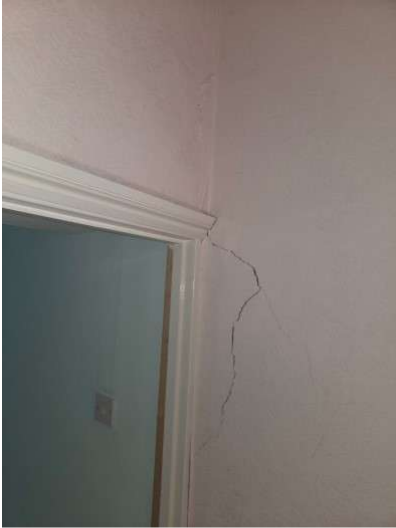
Further illustration of the right hand side party wall to the stair area.
