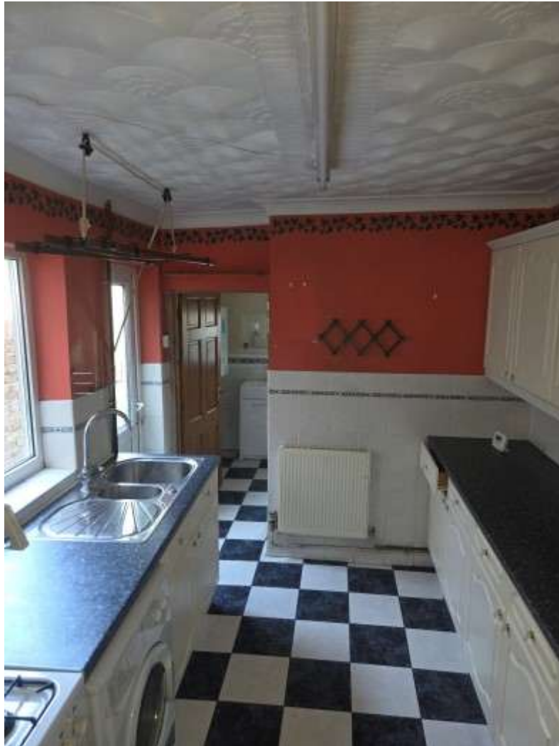
General condition of kitchen accommodation as viewed towards the rear. The photograph shows sloping and distortion of the ceiling. This is particularly apparent towards the rear left hand side of the kitchen where extending towards the bathroom.
