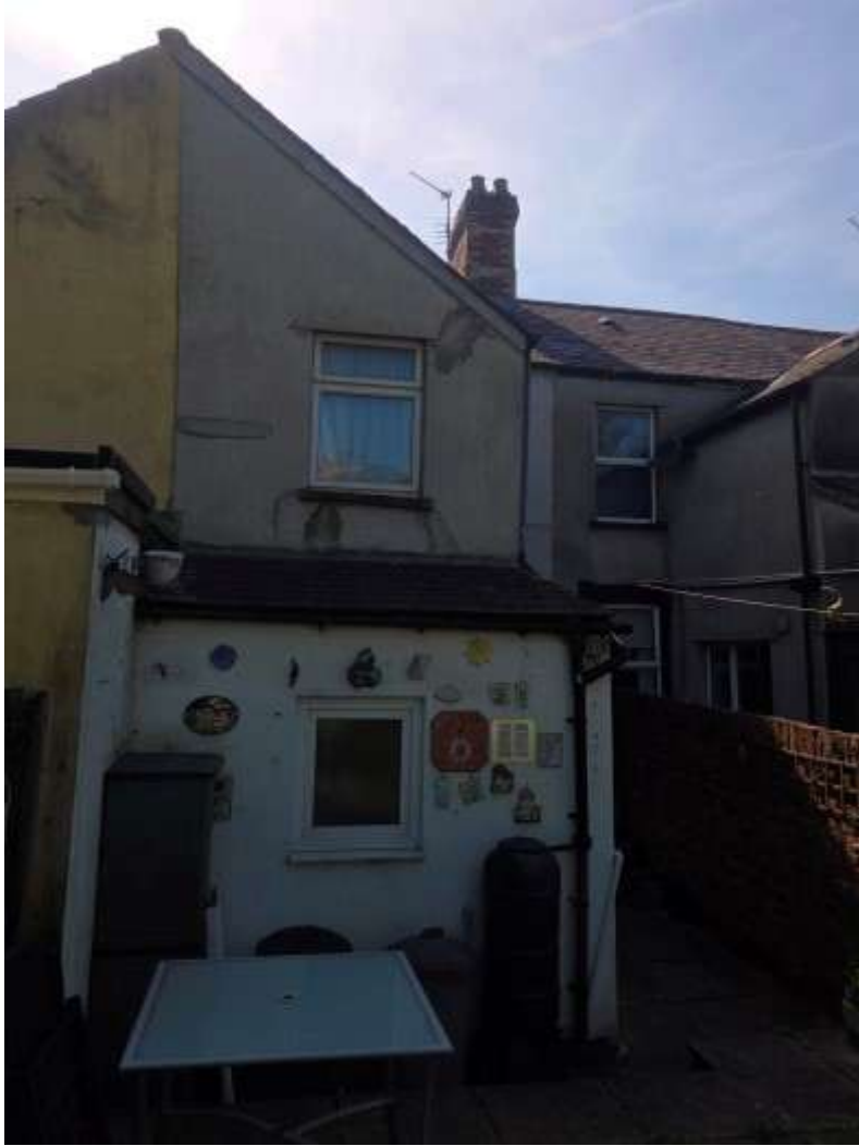
Rear elevation. The photograph shows the walling to the first floor to the rear of the annexe. Areas of past repair in respect of cracking are noted.
