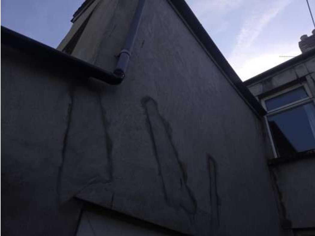
Left hand side wall of the annexe. The photograph shows the render finishes with localised repair noted.
