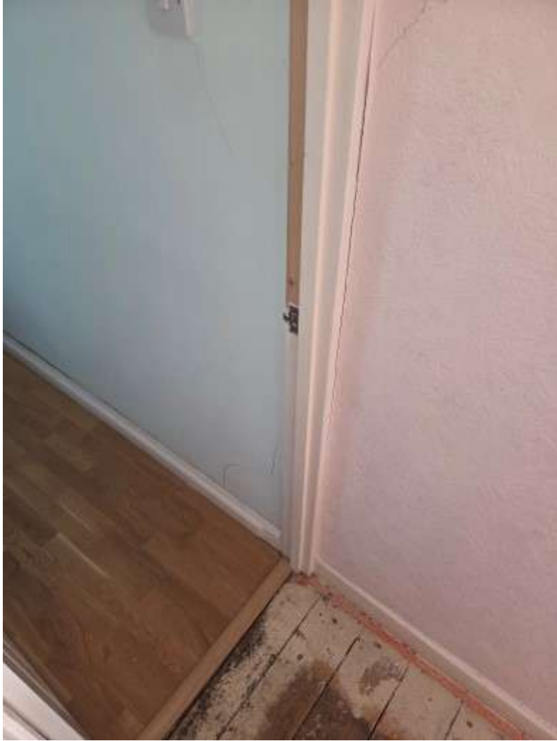
First floor stair/landing area. There is cracking to the right hand side party wall around the door lining to the rear annexe bedroom.
