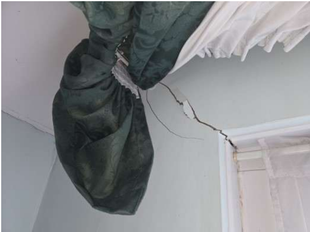
Cracking to the head of the rear annexe bedroom. There is evidence of past repair and replastering work having been carried out with cracking having subsequently reopened.
