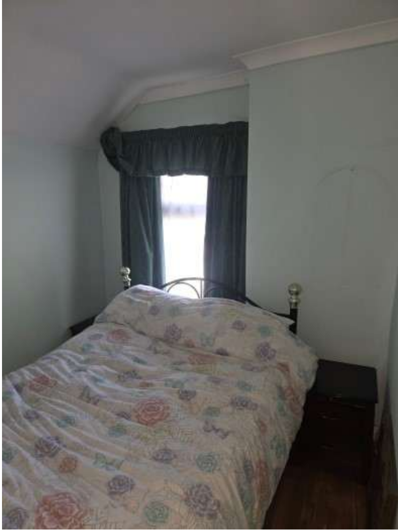
Rear annexe bedroom. There is sloping of the floor from right to left.
