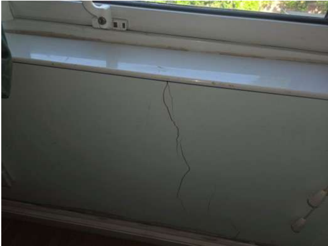
Cracking below the window opening to the rear annexe bedroom.
