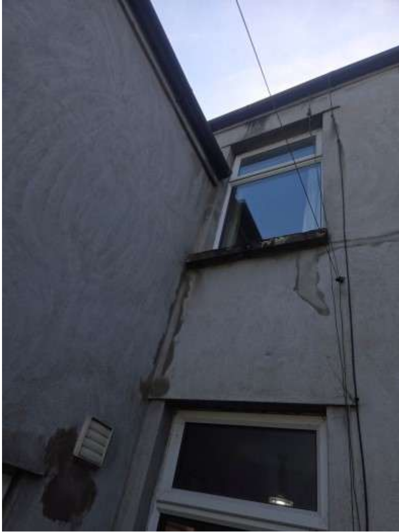
Rear wall of main building. The photograph shows the render finishes. Localised area of repair in respect of cracking is noted.
