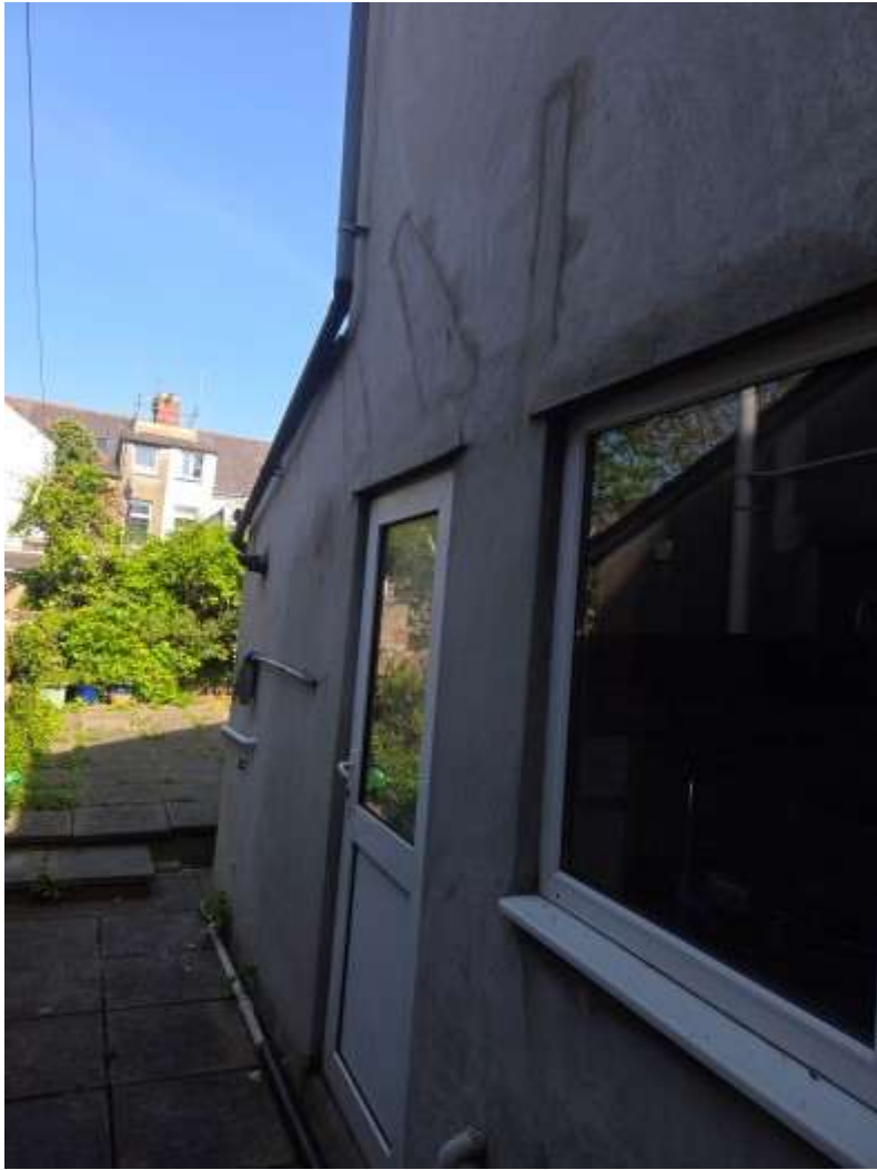
Further illustration of walling where extending to the side of the annexe and to the rear single storey bathroom addition.
