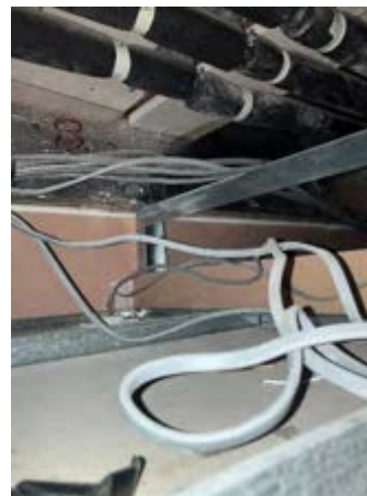
Cable and pipe penetrations to compartment wall
