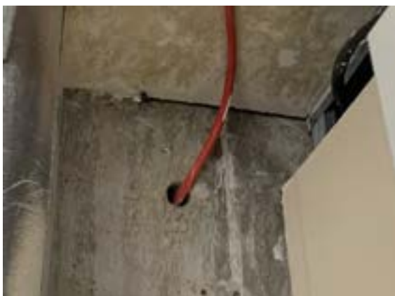
Potentially Inadequate Fire Stopping
