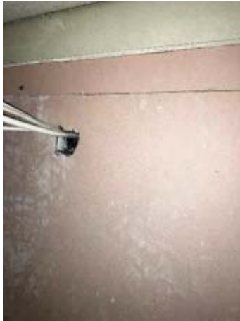
Cable penetration to compartment wall
