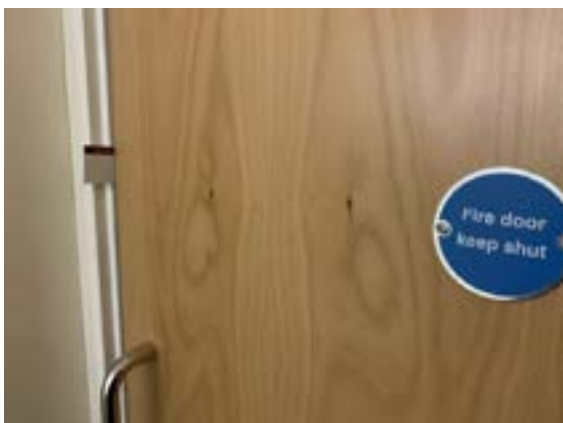
Excessive FD Gap
