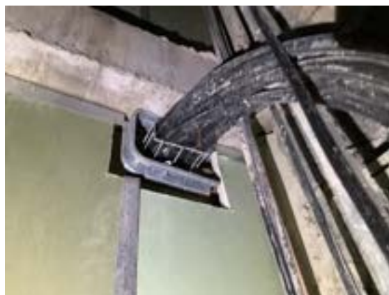
Potentially Inadequate Fire Stopping
