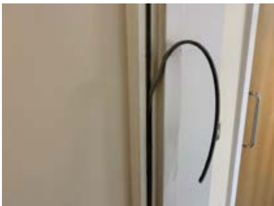
Damaged Intumescent Strip
