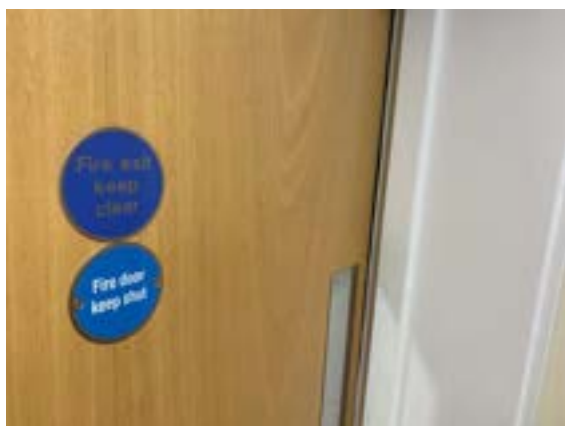
Fire Door - Not closing 100%
