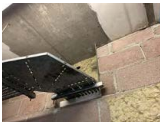
Inadequate Fire Stopping
