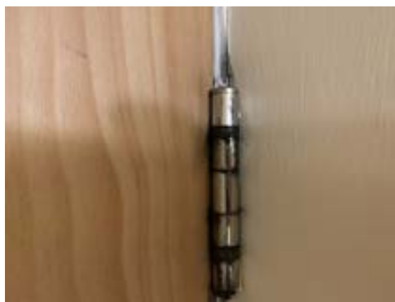
Leaking FD Hinge
