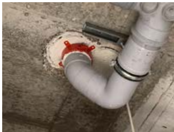
Fire Collar - Not fixed to soffit
