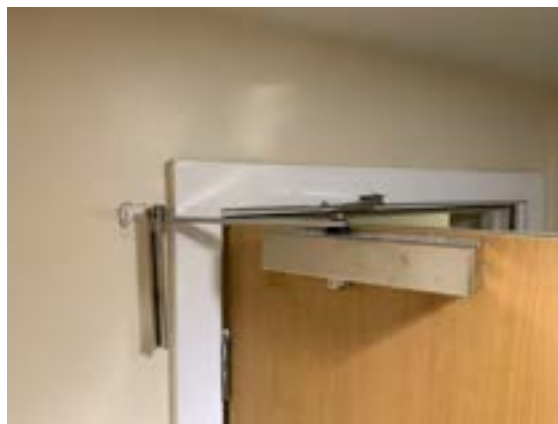
Fire Door - Broken Self-closer
