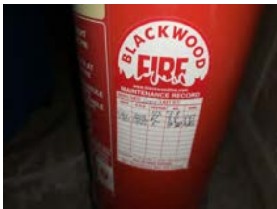
Expired Fire Extinguisher
