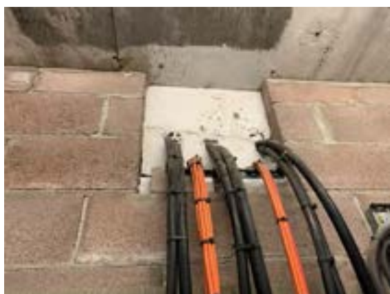
Inadequate Fire Stopping
