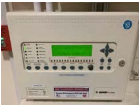
Fire Alarm Panel
