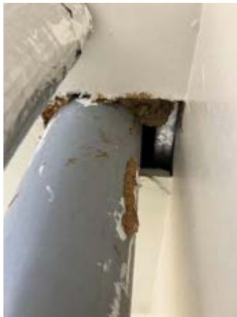
Pipe penetration to compartment floor
