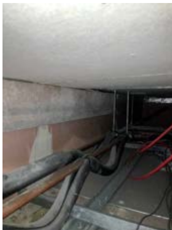
Wall and floor junction not sealed
