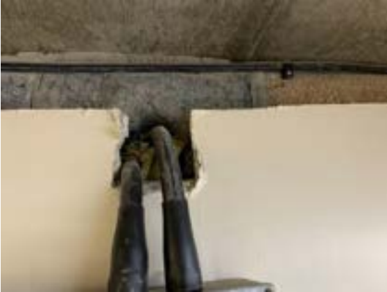
Potentially Inadequate Fire Stopping
