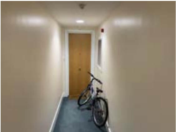
Item(s) in Escape Route
