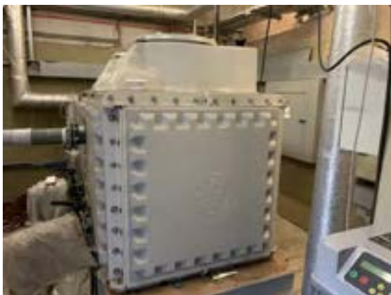
Water Tank Room
