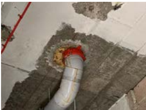
Fire Collar - Not fixed to soffit
