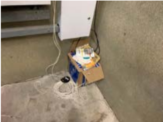
Items in Electrical Intake Room
