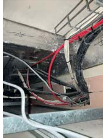
Cable penetration and no fire stopping to compartment wall
