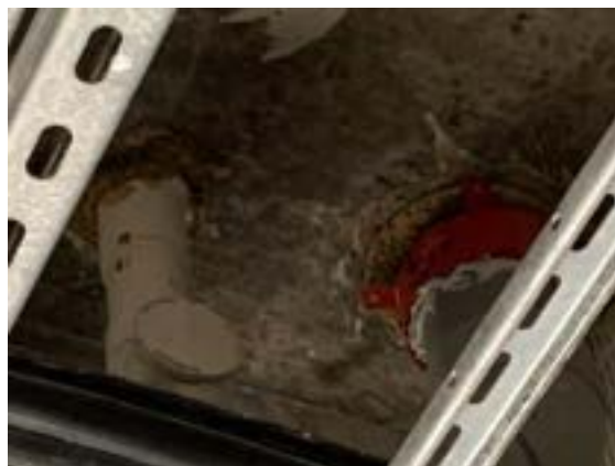
Fire Collar - Not fixed to soffit
