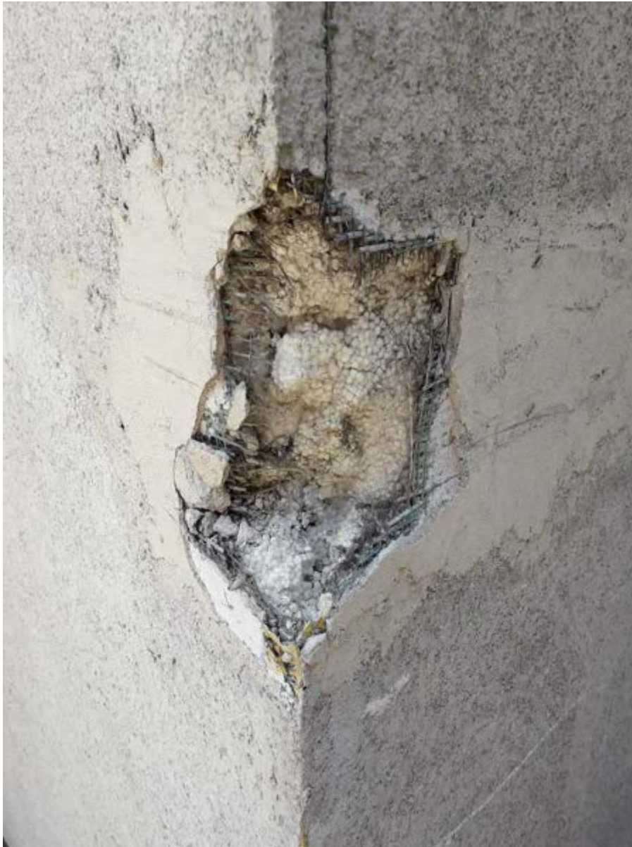
Figure 3 – Photo of damaged corner of render exposing EPS insulation.
