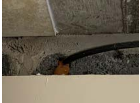
Potentially Inadequate Fire Stopping
